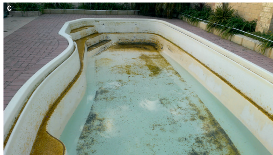
A. Filling the new pond with gravel; a big task, but with big rewards. B,C. Before - a disused pool ready for conversion into a pond. D. The completed pond.
